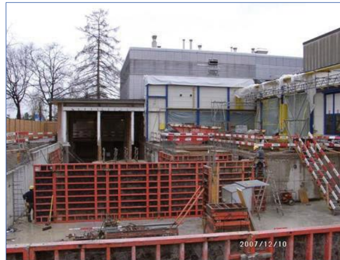
Construction site in December 2007: The new engine test bench will be installed in the new annex building (left).
