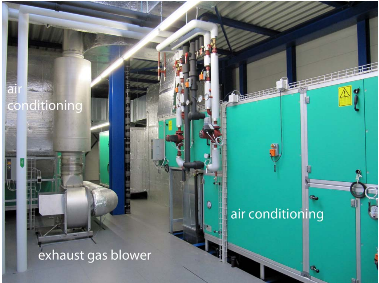
Picture 3: Technique room above test cell
