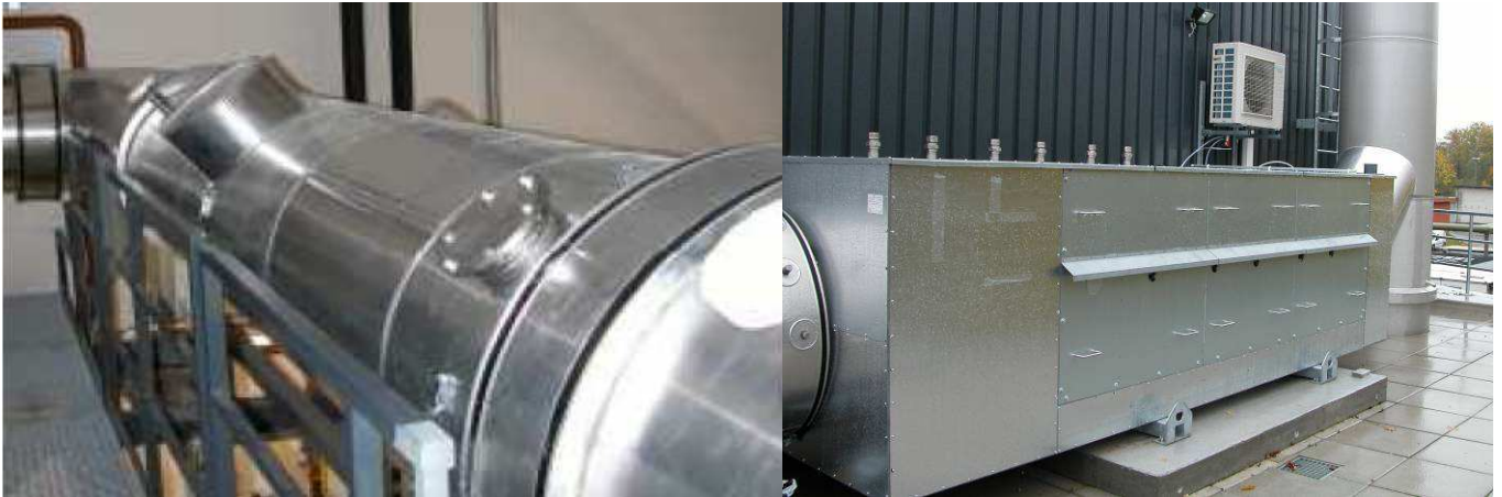
Fig. 3: Exhaust gas after treatment: Long mixing length for Urea vaporization (left) and outside placement of large catalytic converter before treated gas leaves through the chimney in the background (right).
