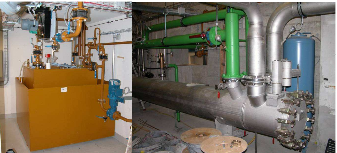
Fig. 2: Day tank and Aare water heat exchanger
